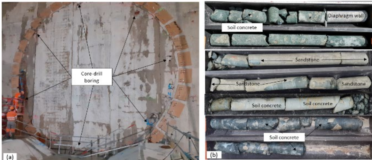
Figure 12. (a) final control before TBM arrival in a shaft; (b) horizontal core-drilling for a gallery.
